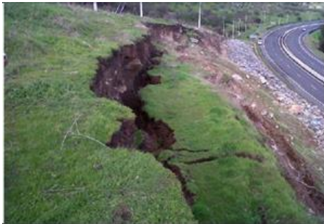
Figure 2. Slope failure registered in August 2013
