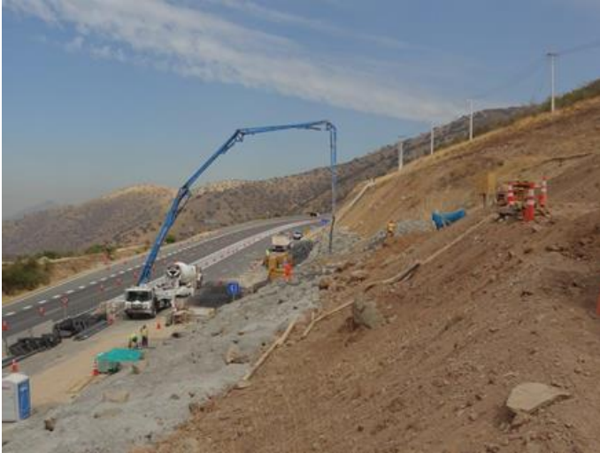
Figure 11. Execution of the concreted rockfill wall at the toe of the slope
