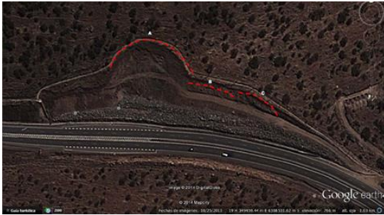
Figure 1. General view of the stabilization measures constructed in 2009 (laying down of the slope inclination and rockfill wall reinforcement)
