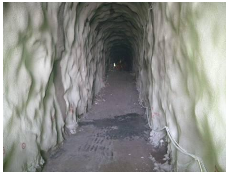
Photo 9. Rock Trap at Tinguiririca Tunnel
