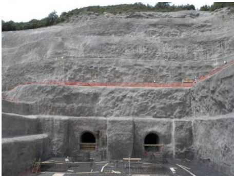
Photo 7. Power-house. Manifolds portals
